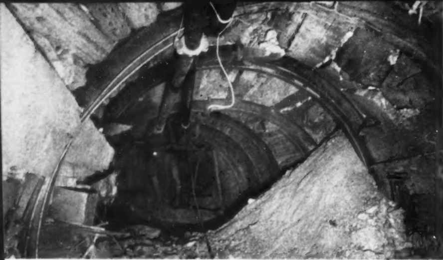
Miami Copper Company now uses 6½-foot diameter circular steel sets spanned with three-inch lagging to support slusher drifts in its revised block caving system. Though the easily-replaced lagging bells out and breaks by the weight developed, the set remains, by and large, unharmed.
